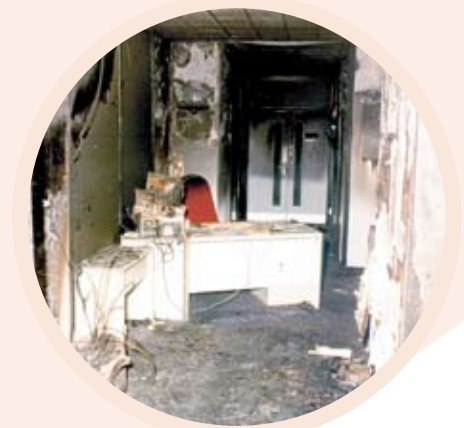
The result of an office fire
